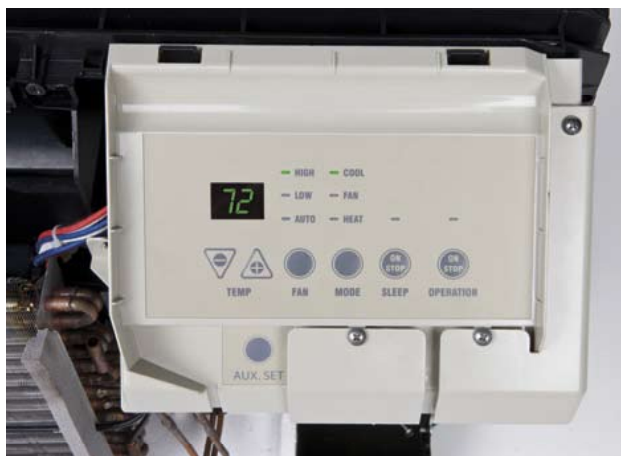
Enclosure cover removed.
