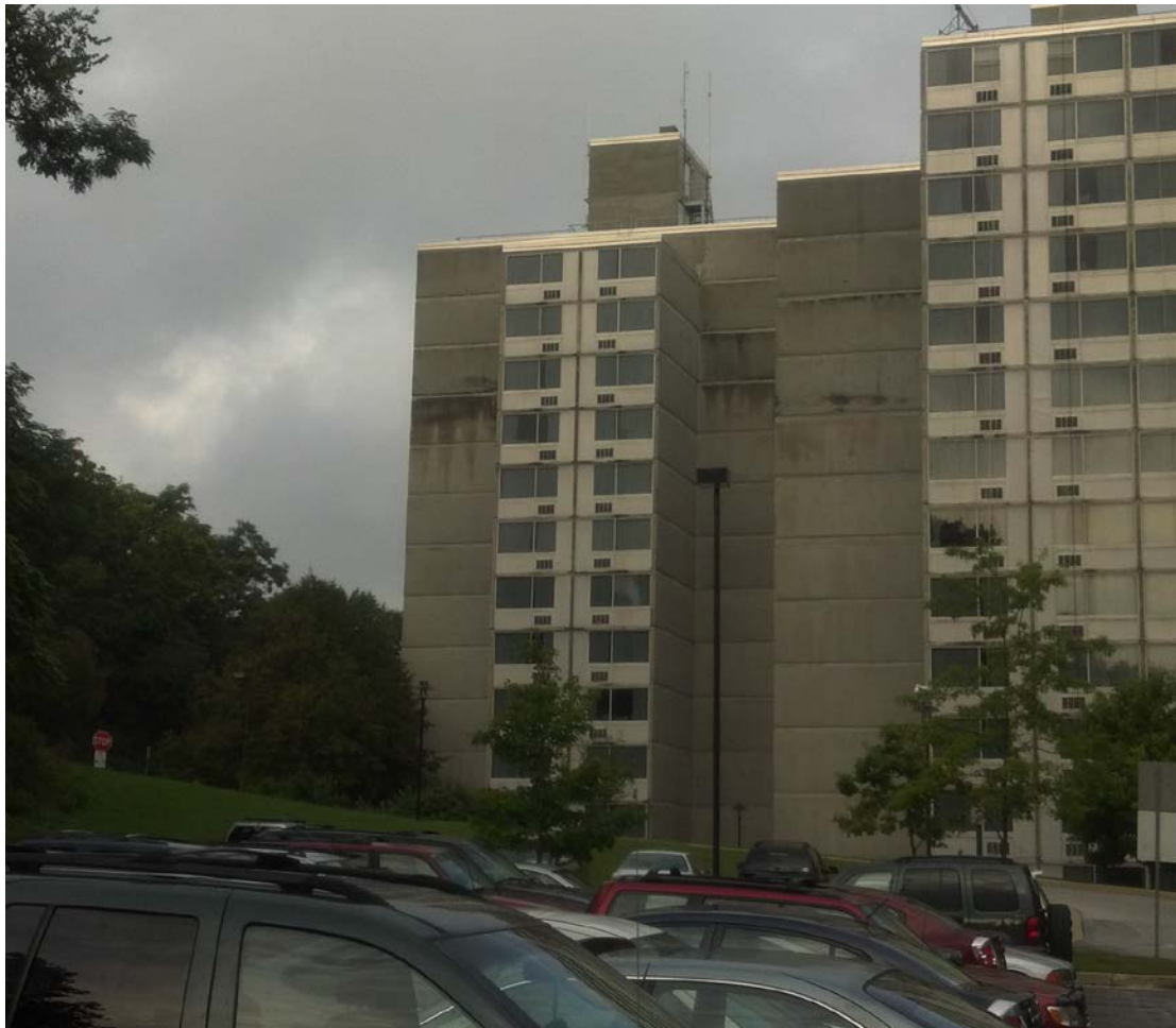
Figure 3 – Concrete staining from rain
